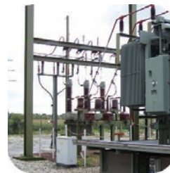
Power Transmission and Distribution
