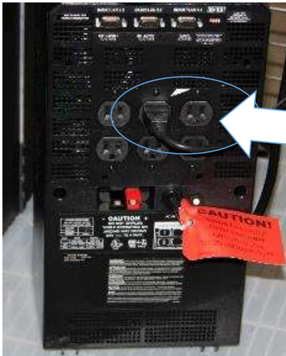
Back of UPS with printer power cord plugged in
