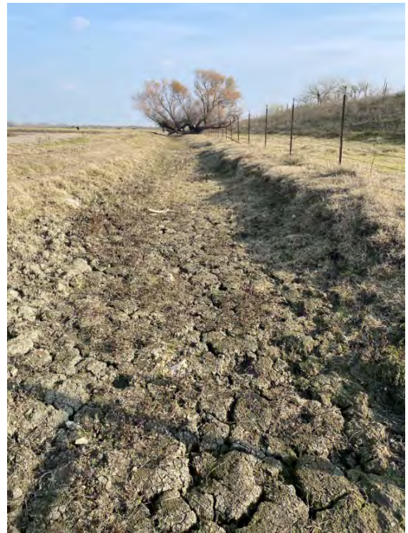
Ephemerally inundated Ditch (107.1) located in the southern edge of Field 3 at the Bank.
