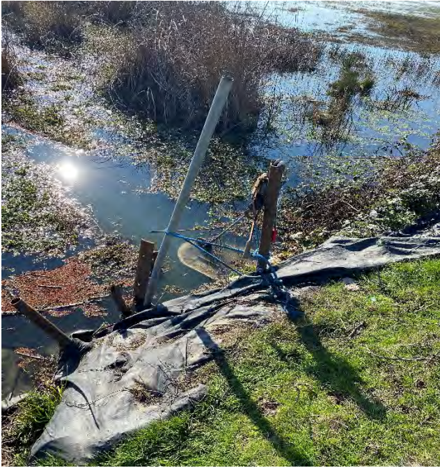
Photograph 5. The out fall culvert from Watson Hollow Slough and in-fall culvert to the wide ditch have gate valves which are operable and are located at the north end of the ditch.
