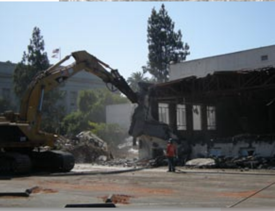
Above: In just a few weeks, crews demolished the former Administrative Annex and established a grassy park area in downtown Fairfield. Top: A conceptual drawing of the William J. Carroll Government Center planned for construction in Vacaville.
